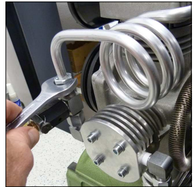
Fig. 1 - Loosen pipe connections
