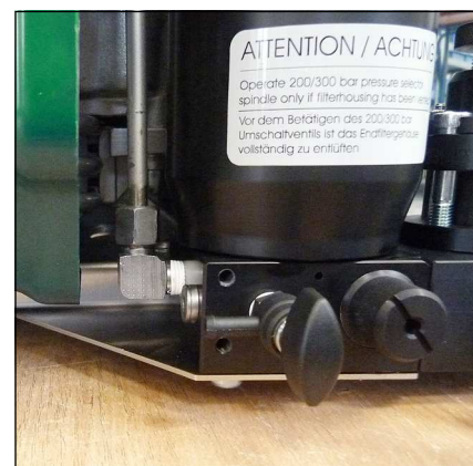
Fig. 2 - Condensate drain valve 3.stage
